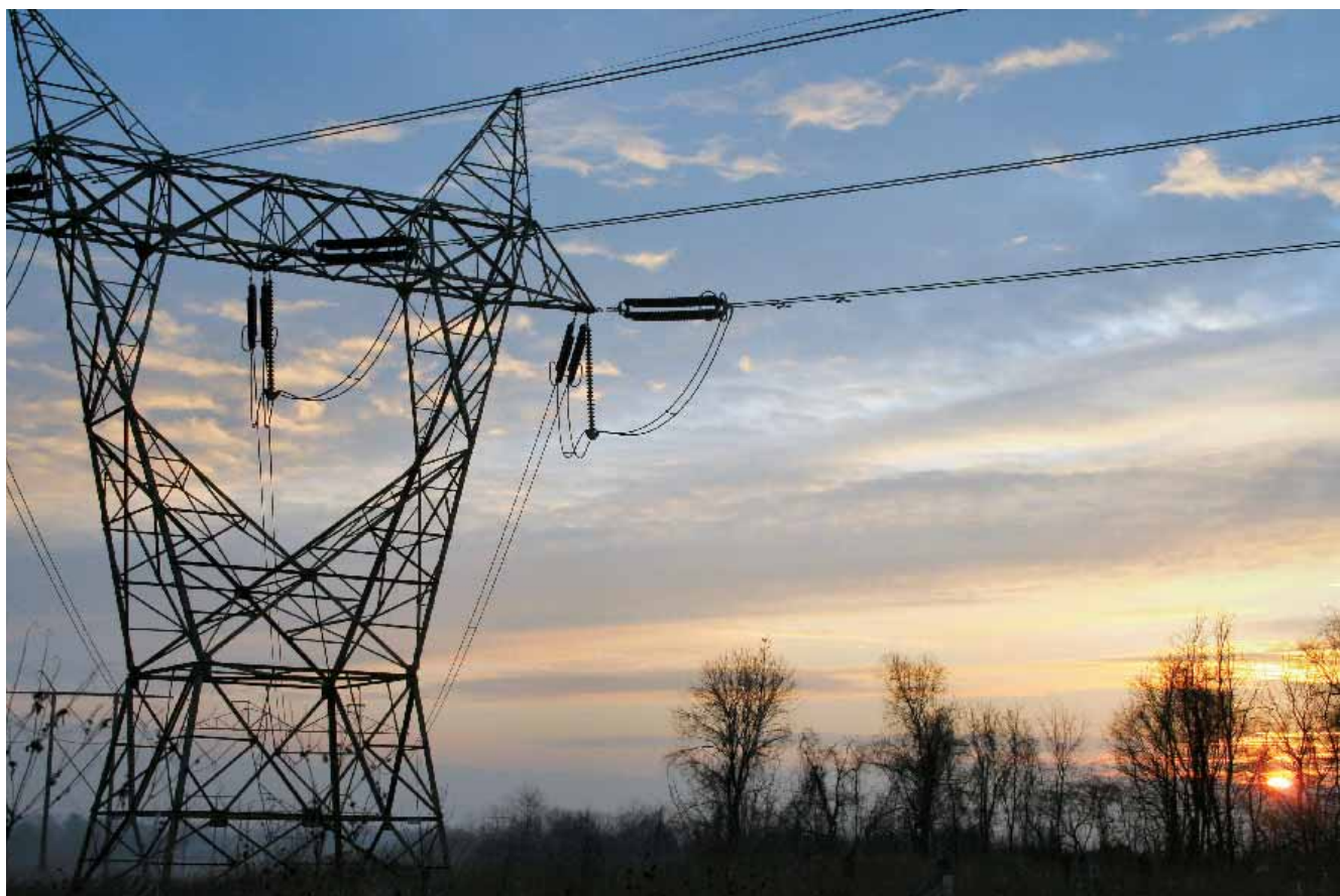
ASSURED POWER: The transmission sector has also been opened up and nearly a score of private players are entering the business
